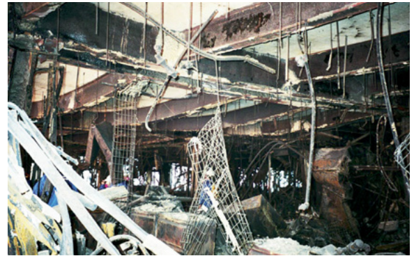
Fire damage in WTC 5 (2002 NIST survey of fires that resulted in total or partial collapse).
