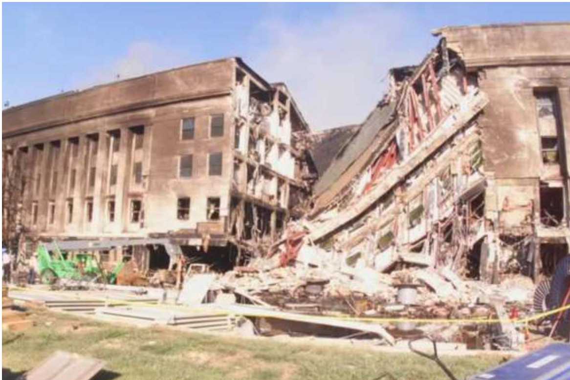
Figure F-8 Warning lights and collapsed section (see red lights at bottom right)
