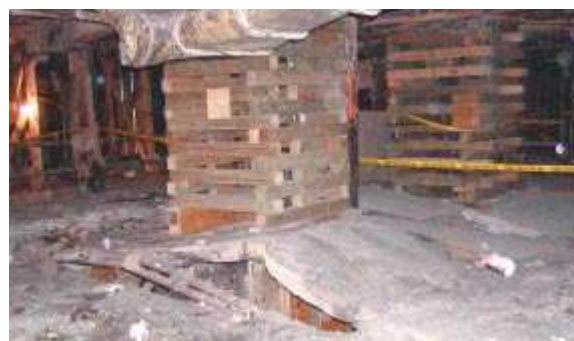
Figure H-2 Pentagon Building and Performance Report Figure 5.27 Breached second-floor slab
