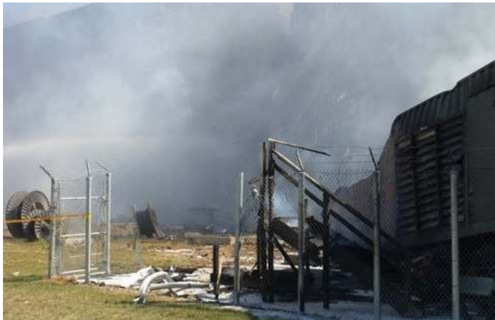
Figure F-4 Generator trailer and fence The north end of the trailer is gouged
